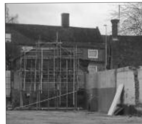
Site of the Old Depot taken from Magdalen Street, showing rear of the remaining frontage in Military Road
