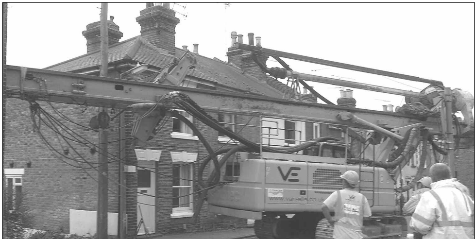
The problems caused by too large vehicles and too narrow streets
